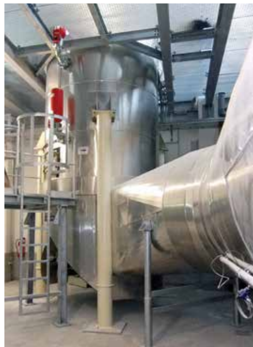
Dryer lower section with drying air inlet
